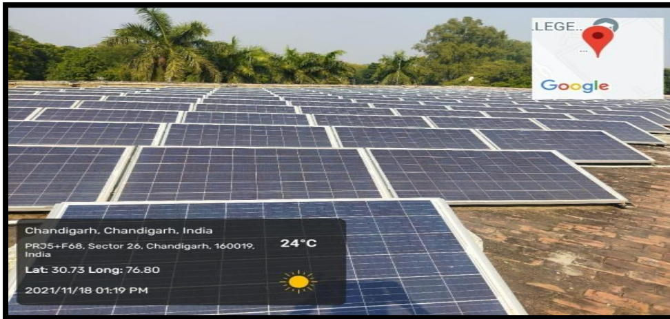
Solar Panels on the rooftop of Boys Hostel of the College
